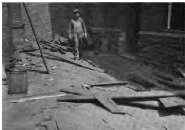
Fig. 3. Poor "Housekeeping" Conditions.‡
